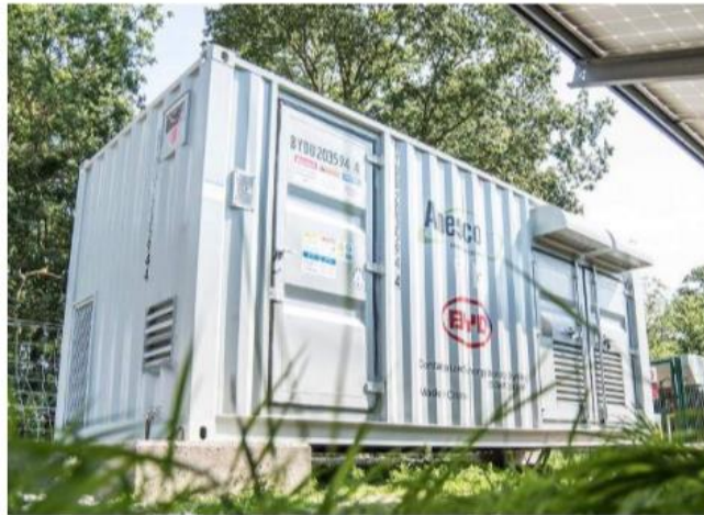
Forty containers, each containing a battery, have been proposed for land off Broadway Lane.
